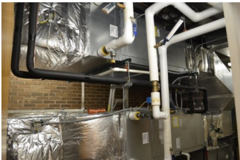
Air Handlers – One for each floor
