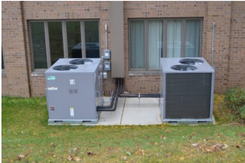
Outside AC Compressors – One for each Floor
